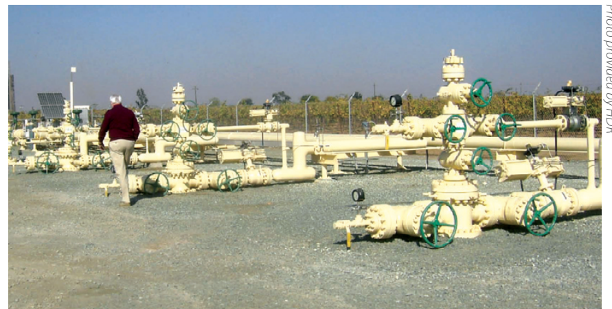
Above: A wellhead site.
